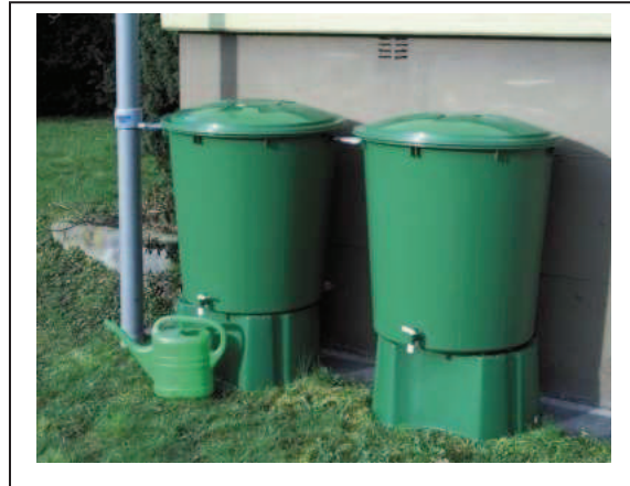
Figure 1. Plastic tanks (ground level)
