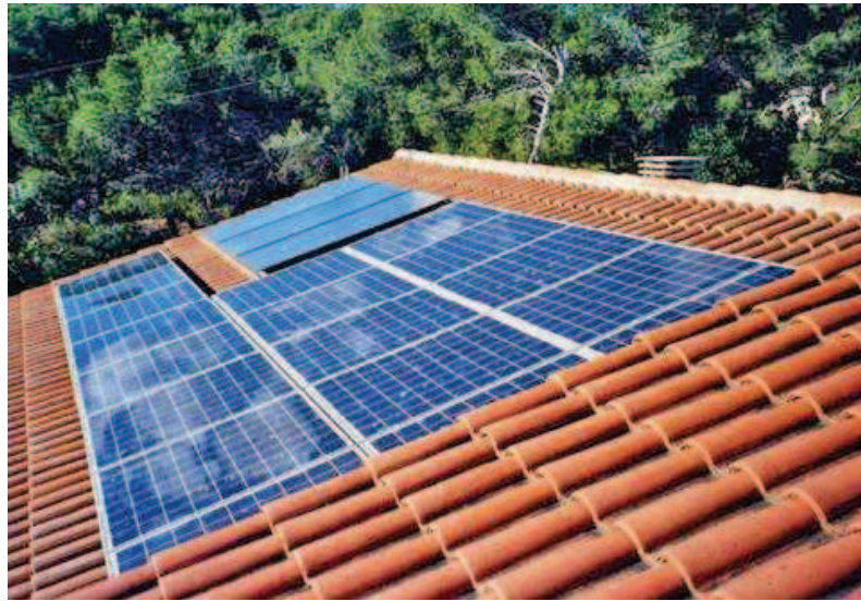
Illustration 2 Installed photovoltaic panels
