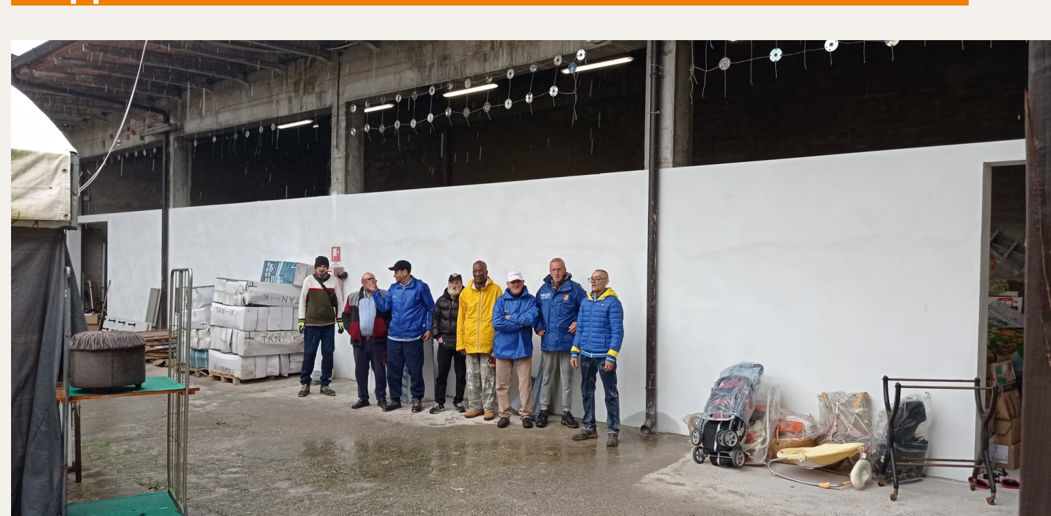
Companions at Piadena pose in front of the warehouse under renovation. - Credit: Emmaus Piadena
